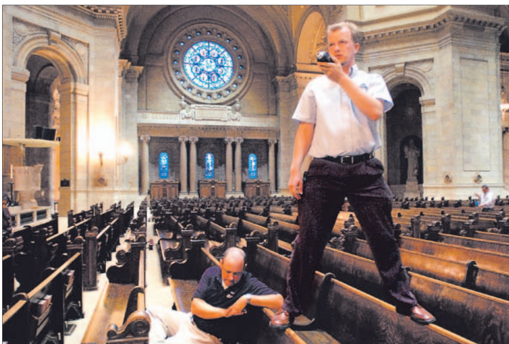
BRANDI JADE THOMAS, PIONEER PRESS Standing atop pews, Stefan Svärd uses a meter to take sound-level readings as he works on the installation of a digital speaker system in the Cathedral of St. Paul, whose cavernous space presents an acoustical challenge. Svärd was assisted by Art Gonzales, seated.
